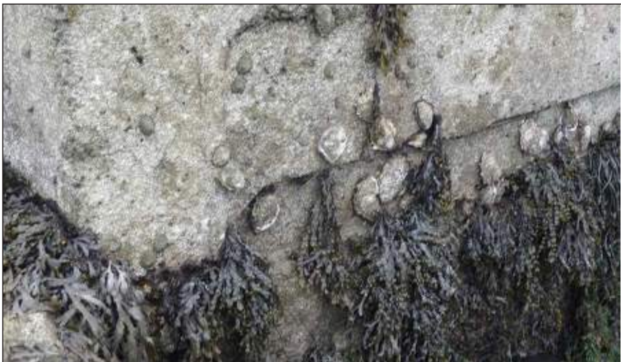
Fig. 219 Pier wall with Pacific oysters.
